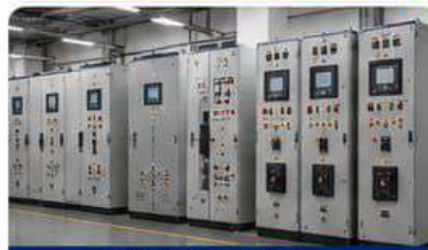
SWITCHGEAR & CONTROL EQUIPMENT
